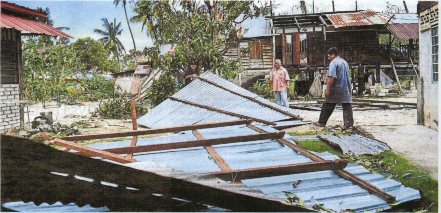
Villagers at Kampung Permatang Pasir check the damage caused by the freak storm. — Picture by Sayuti Zainudin
